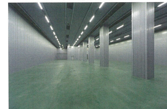
1階コア冷蔵保管庫
